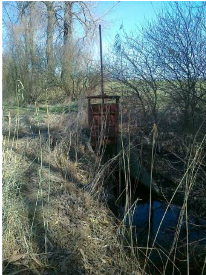
Phot. 1. Neglected drainage system
