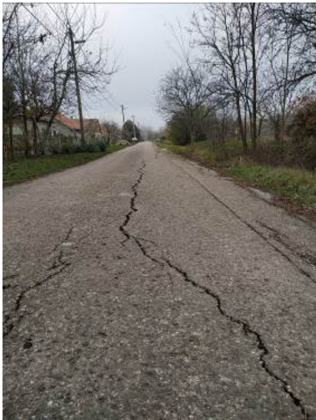
Appendix Figure 6.6 Road in need of repair in Derekegyház
