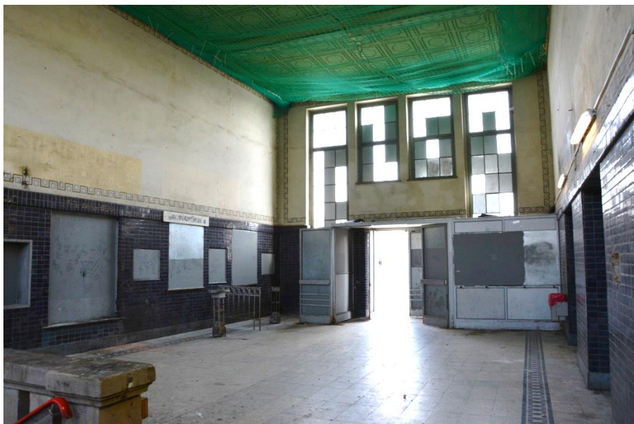
Photograph 5: Train station Erndtebrück; highly decrepited building, now under reconstruction
