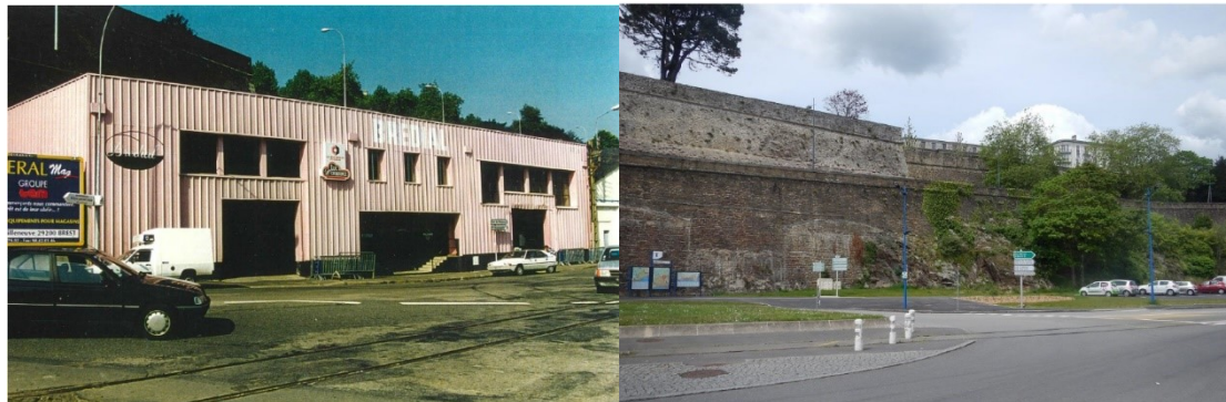
Figure 6.4 Before and after pictures of the deconstruction of a brownfield to clear the view of the Vauban city walls.
